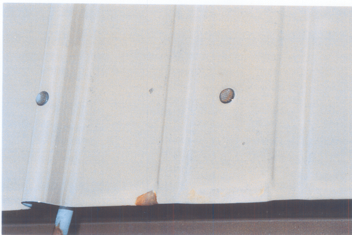
Figure 13b. 11 year old, G-90 Galvanized, Plastisol Paint System, Complex Oxide Pretreatment
