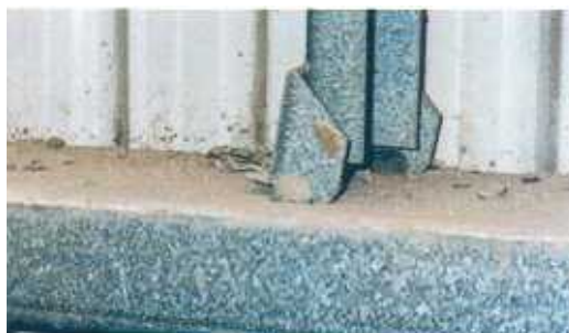
Figure 2: Build-up on purlin
