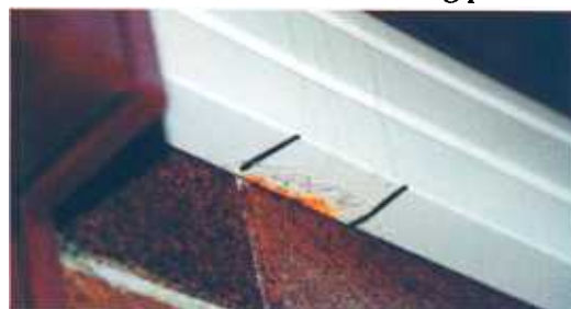
Figure 1: Example of corrosion caused by incorrect acid brick cleaning practices.
