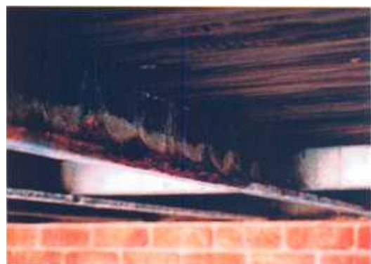
Figure 3: Example of Corrosion that results from contact of CCA Treated Timber with Galvanized Purlins
